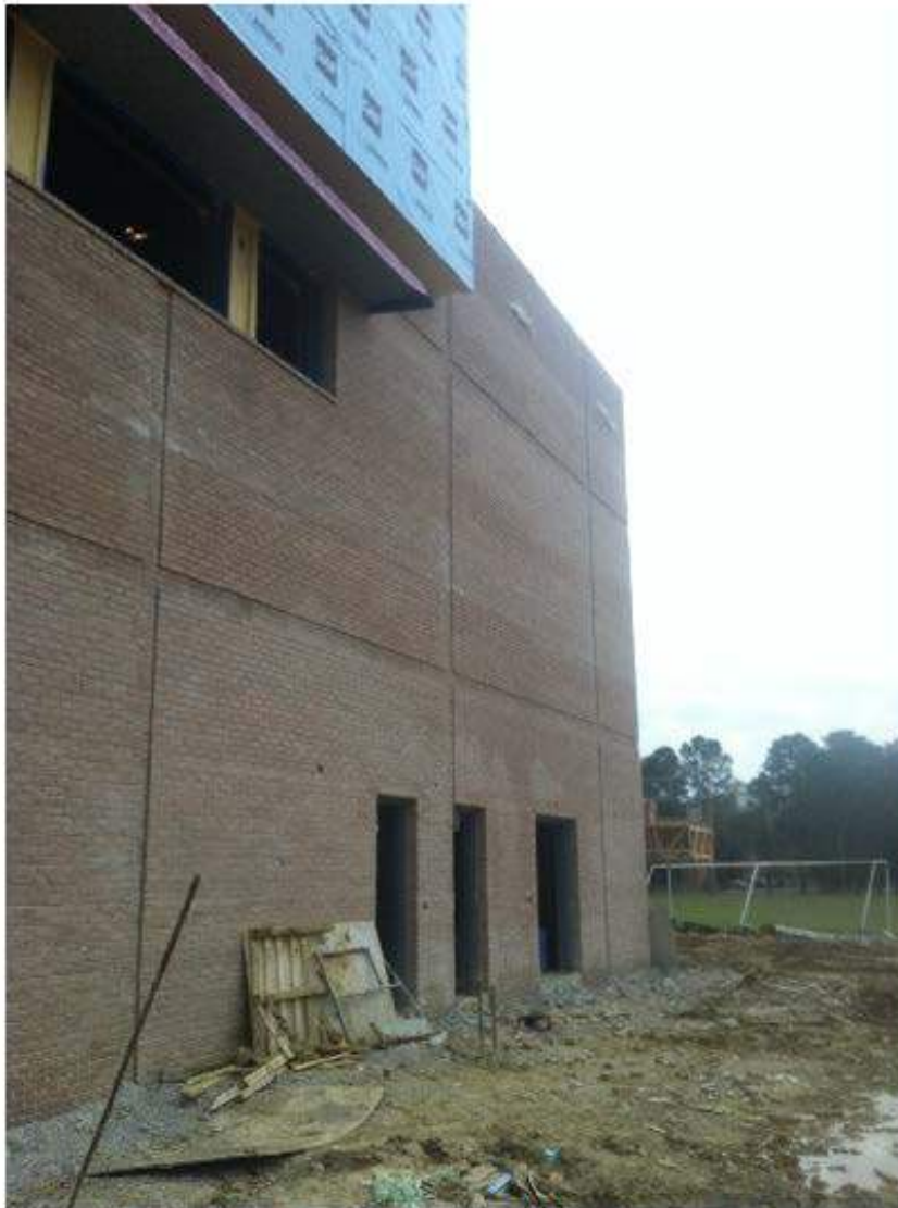
Looking south on the west side toward the future Library Loading Dock.
