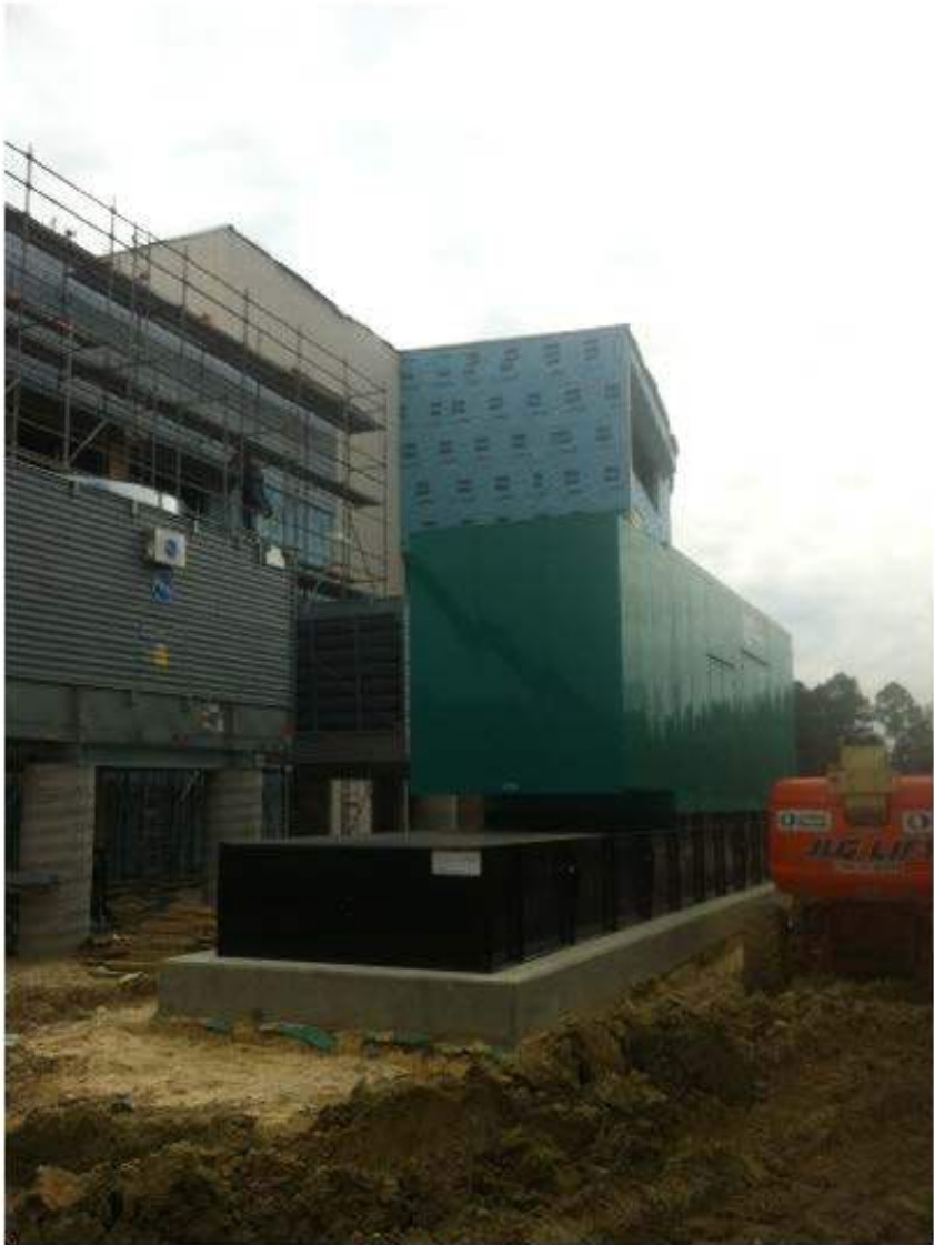
Looking at the green generator.
