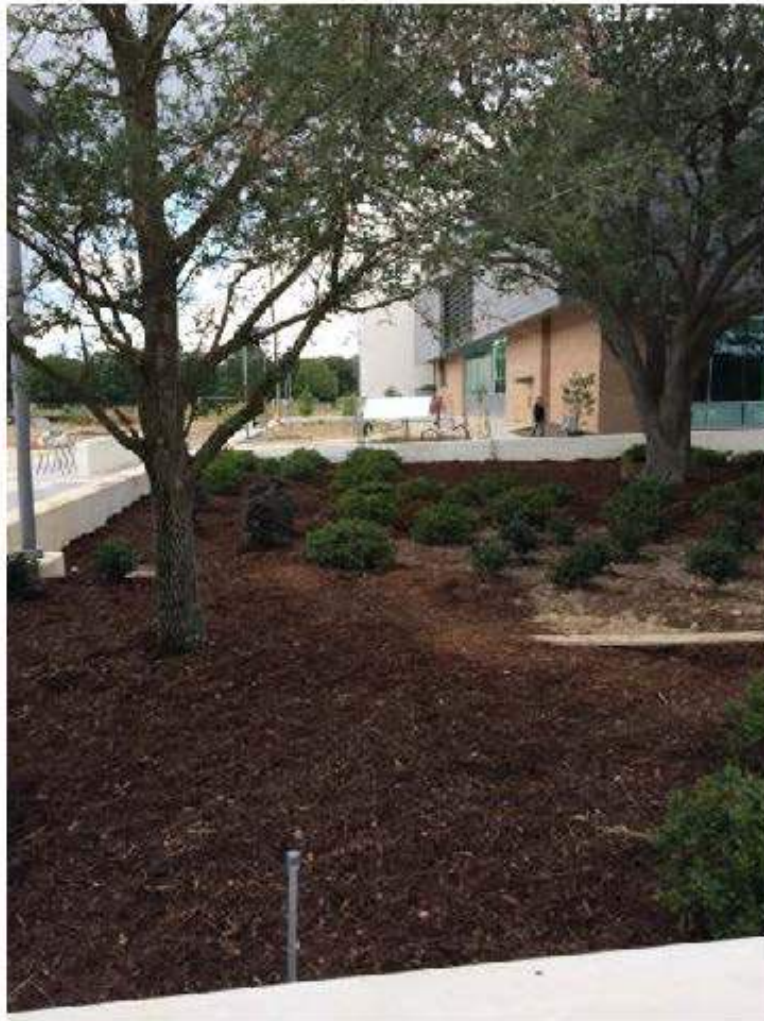
Looking at the bed preparation of the western planting area south of the Plaza.
