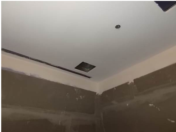
Exhaust fan openings in ceiling of Women 108 and Men 109 not protected.
