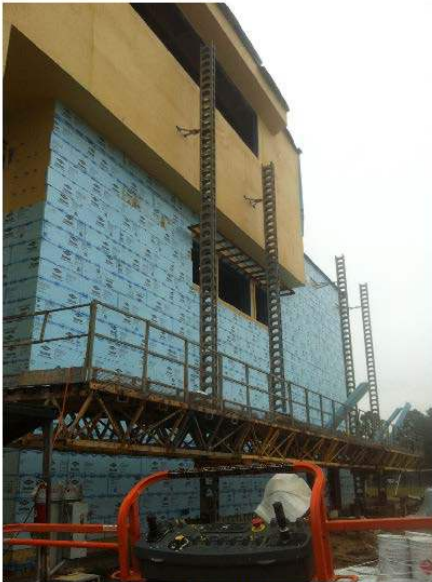
The masonry scaffolding has been installed on the west side of the Library.
