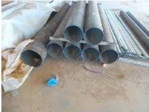
Protect stored materials. Clean out pipe before installation. Also see next picture.
