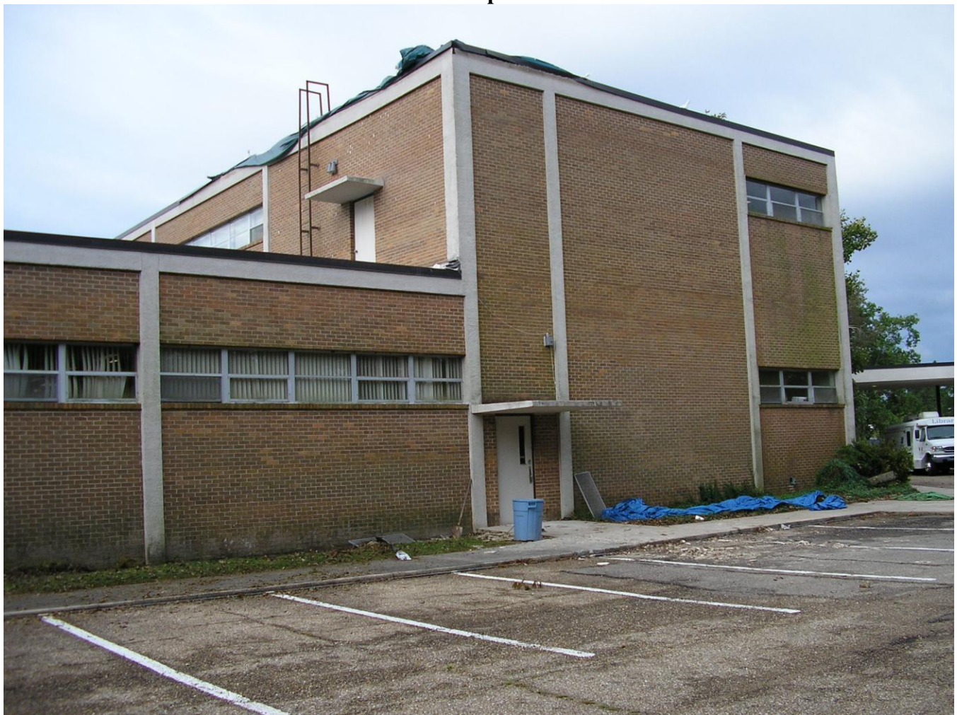
Wind from Ike Blowing Tarp on Corner of Building 9/12/08
