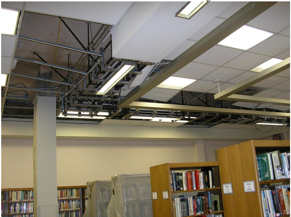
Ceiling Damage on First Floor 9/9/08
