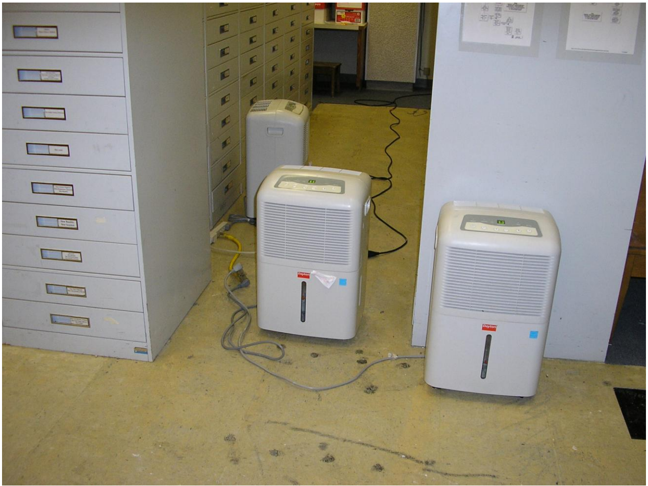
Dehumidifiers Running in Periodicals Storage Room 9/12/08
