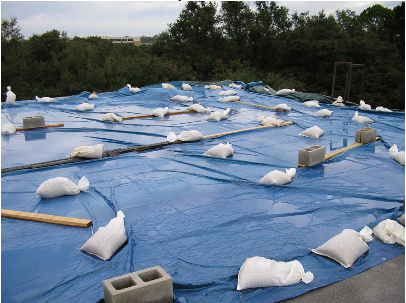
Sand Bags and Cinder Blocks Holding Down Blue Tarp on Roof 9/12/08
