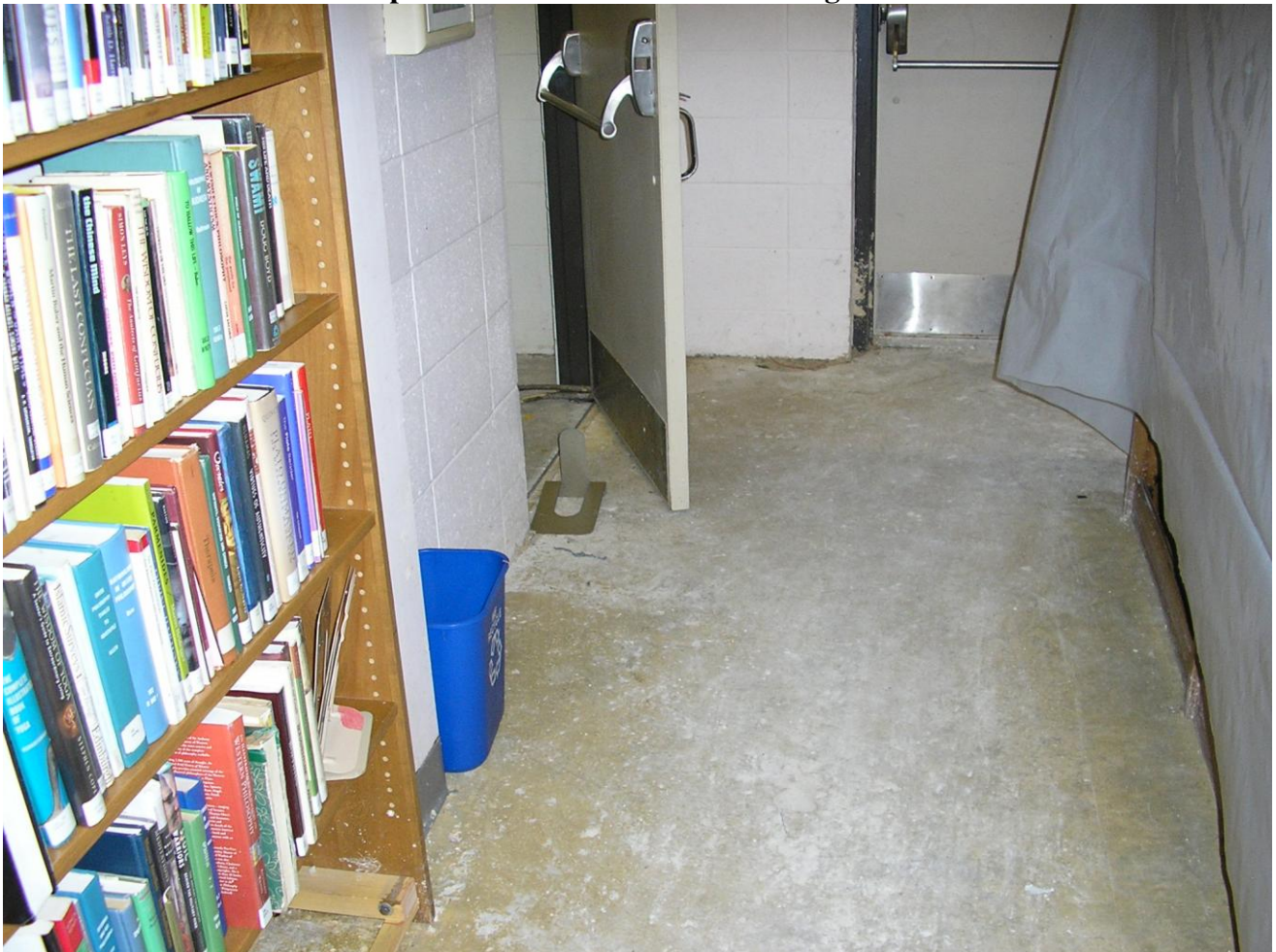
Site of Water Intrusion on First Floor 9/5/08
