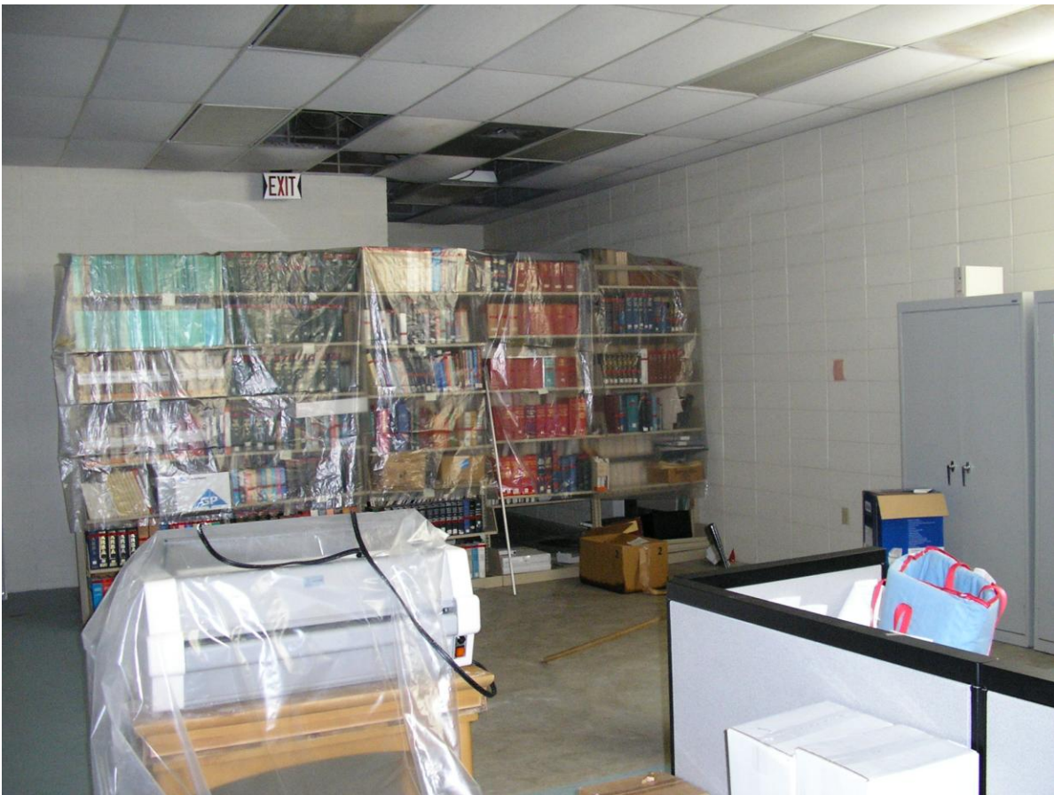
Computer Division under Roof Damage 9/5/08
