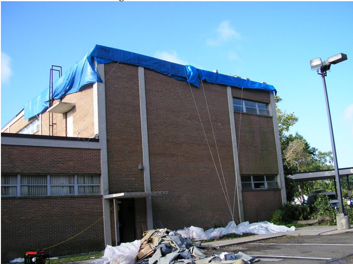
Blue Tarp Over Computer Division Roof-Site of Water Intrusion 9/3/08
