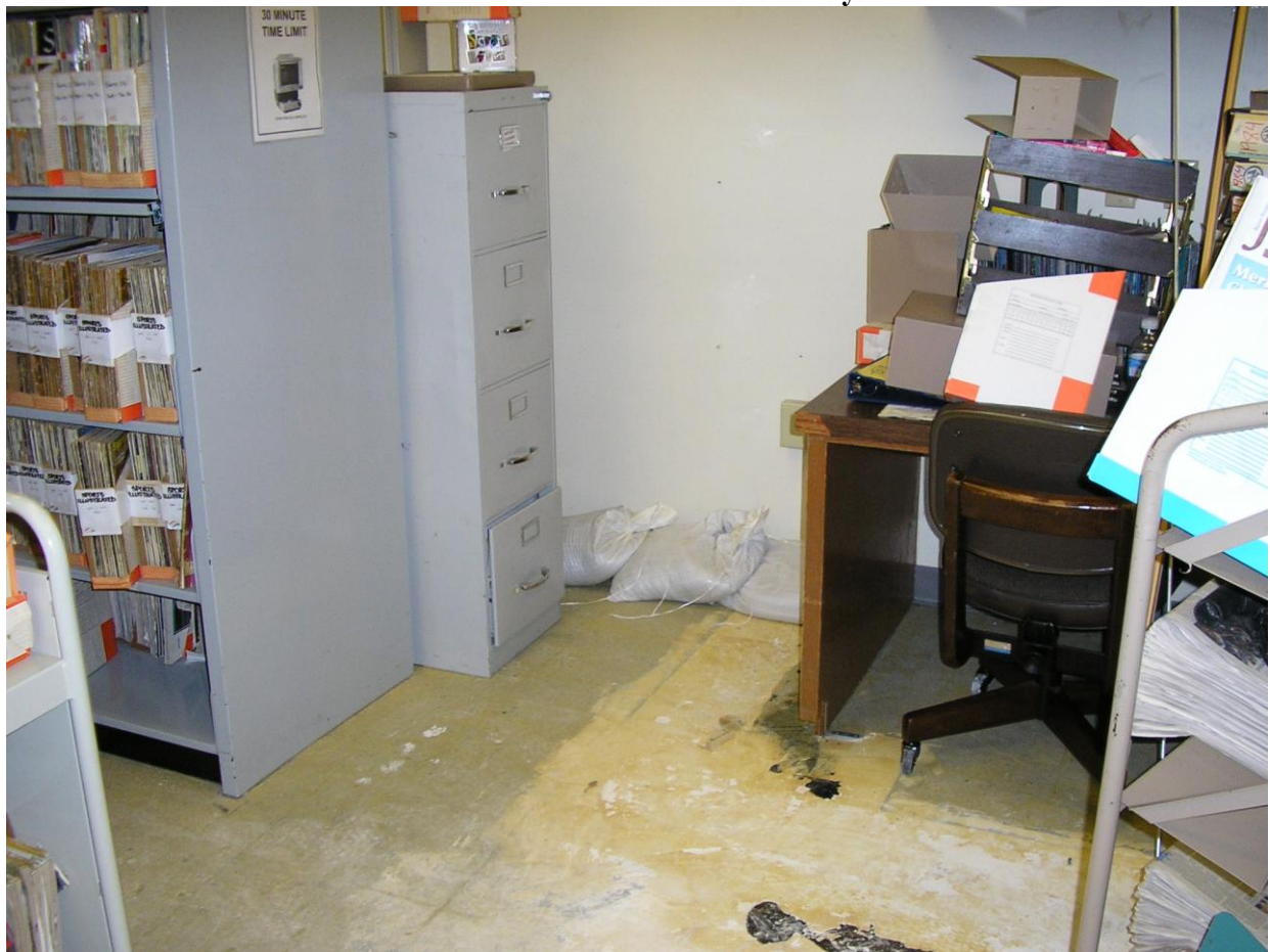
Sand Bags in Periodicals Storage Room 9/12/08
